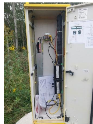
Monitoring station with remote corrosion rate sensor measurement equipment
